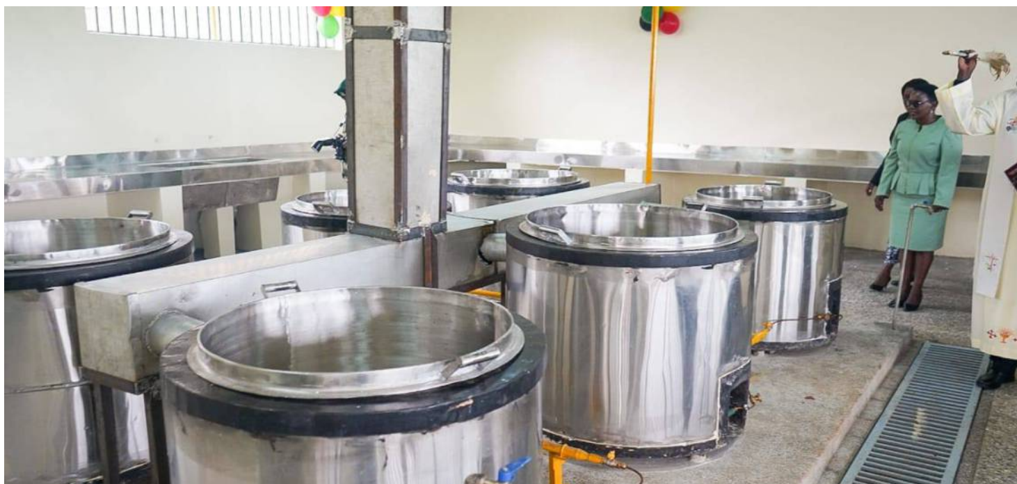
LPG cooking equipment at Lang'ata Women's Maximum Prison, the first facility to fully complete the clean cooking transition
