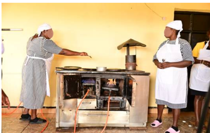
Biogas digester at Embu Women's Prison; converting organic and human waste into clean renewable energy for cooking
